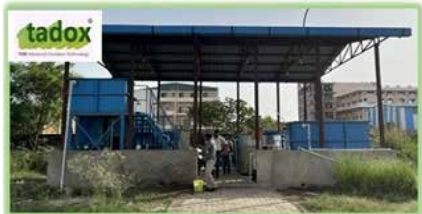
20 KLD TADOX® Plant in Textile CETP in Kanpur; Funded by National Mission for Clean Ganga, MoJS, GoI
